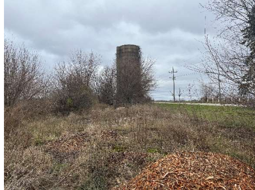
View of Dilapidated Silo at East-Central Property Boundary of 02-19-200-006
